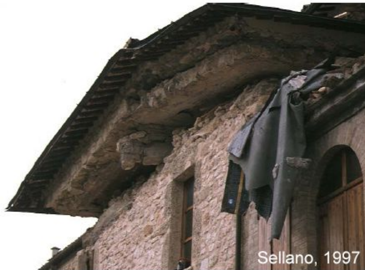
Sliding of the roof floor: the masonry is not adequately strengthened
