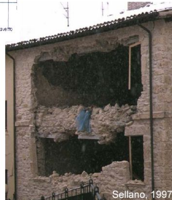
Expulsion of the façade: the tie-beam is supported only by the internal leaf of a multi-leaves masonry: load eccentricity and reduction of the resisting area
