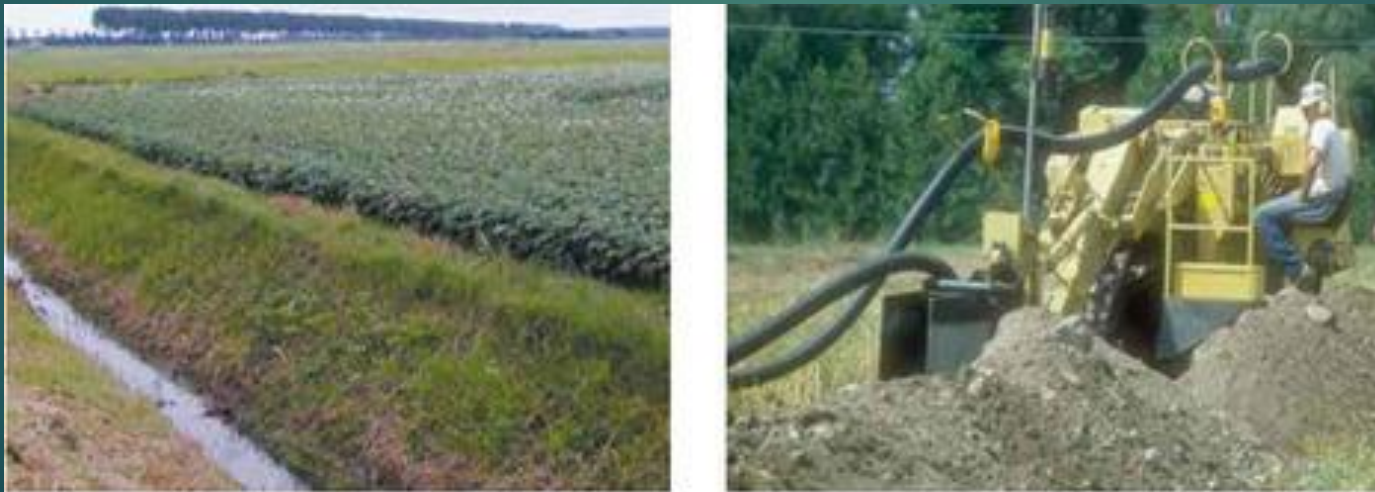
Figure 17.13. Left: Drainage ditch removes excess water and lowers water table. Right: Installation of perforated corrugated PVC drain lines using a laser-guided trencher.
